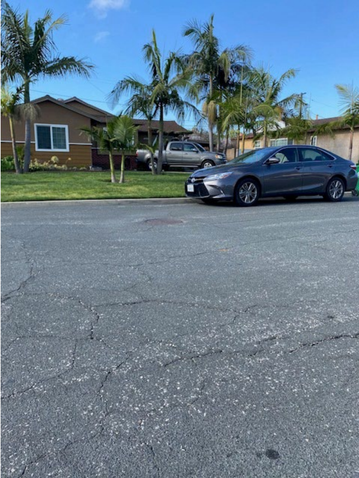
Photo #4 - 04/24/2024 – subside street and subside manhole number 2006 at the intersection of Pembroke Lane and Webber Place (looking south)
