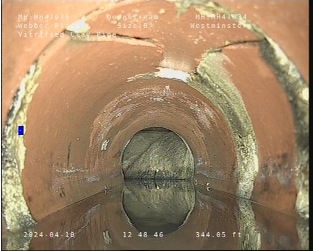
Photo #1 - 04/10/2024 – CCTV photo of a damaged pipe a few feet north of manhole number 2006
