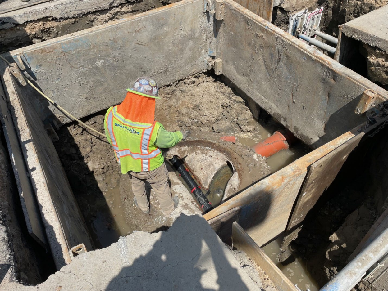
Photo #6 – 05/14/2024 – ground water issue after excavation
