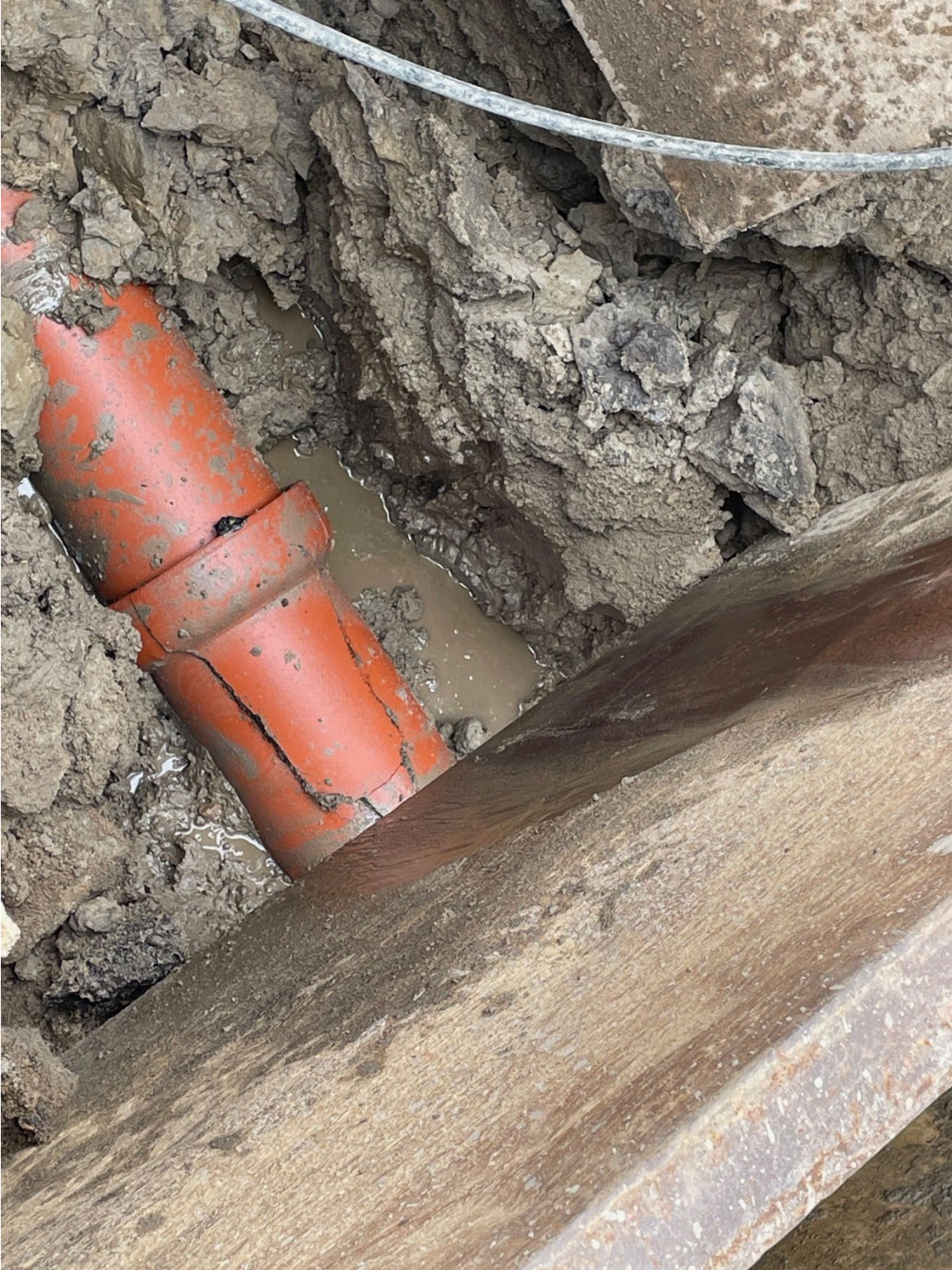
Photo #5 – 05/13/2024 – condition of the broken sewer pipe after excavation
